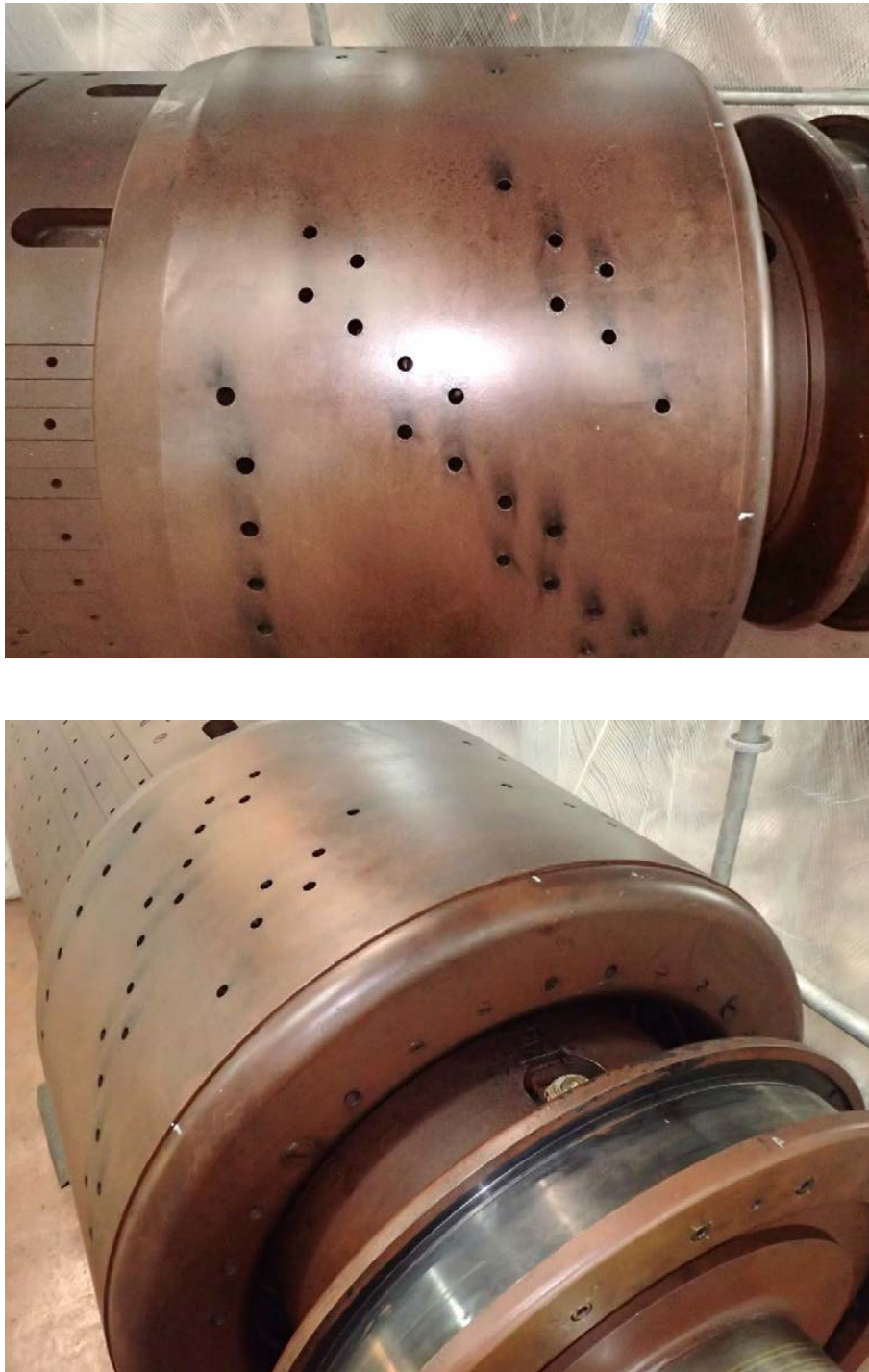
Figure 24. Views of the intact retaining ring and centering ring at the north end of the generator rotor. The pattern of cooling passages in the retaining ring are a result of the positions of end winding components and cooling pathways between or through components inside of the retaining ring. Note that in the lower image, the cooling fan (ring) is near the centering ring , but the blades have been removed.
