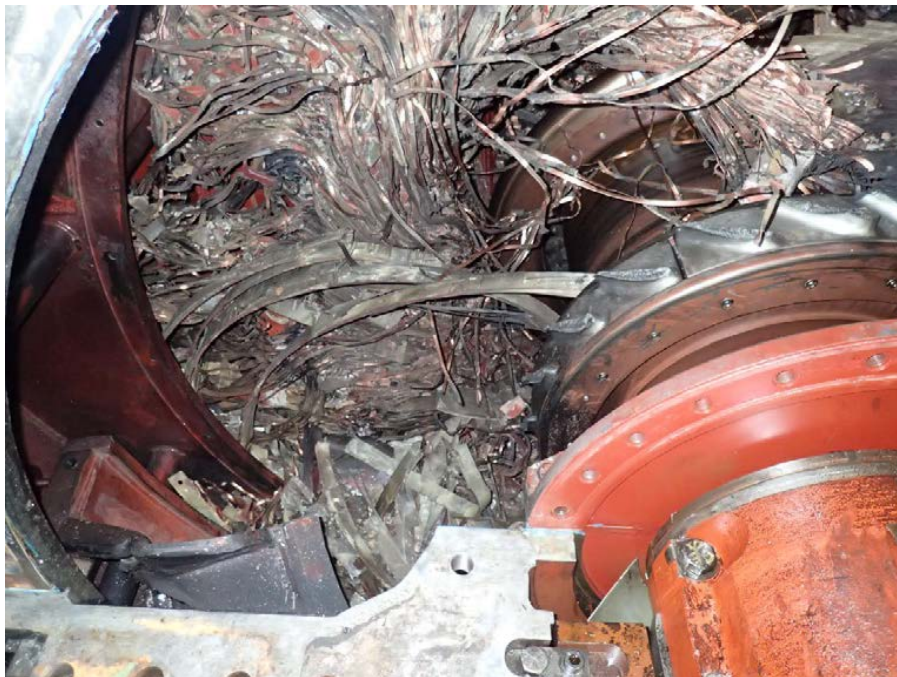
Figure 6. Additional views of the south end of the generator. The upper image shows one of the fractures on the retaining ring (arrow), and the lower image shows damaged windings, broken blades on the hydrogen cooling fan, and other damaged and displaced components.
