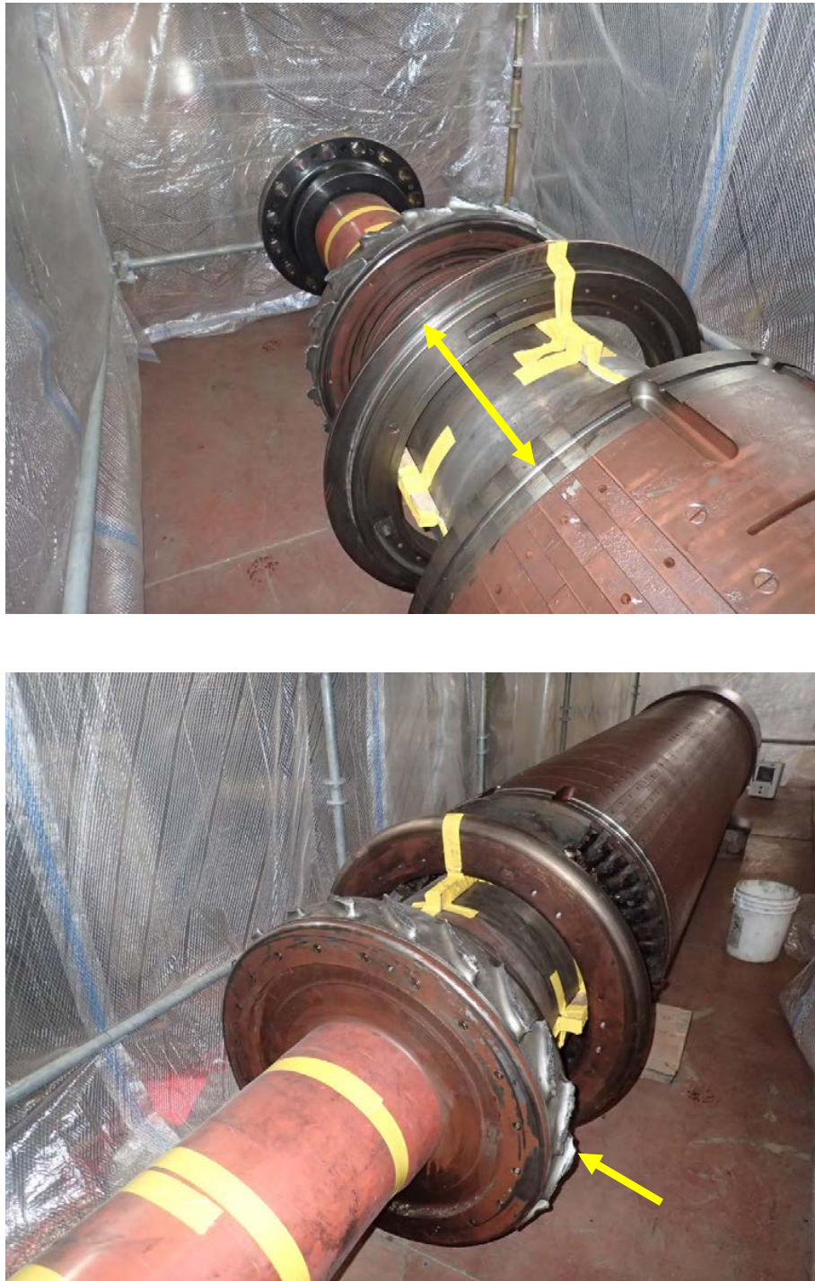
Figure 21. Views of the south end of the generator rotor. The arrow in the upper image indicates the approximate location where the retaining ring was attached, between the centering ring and the end of the rotor, and on the outside of the end windings. The arrow in the lower image shows the location of the hydrogen cooling fan.
