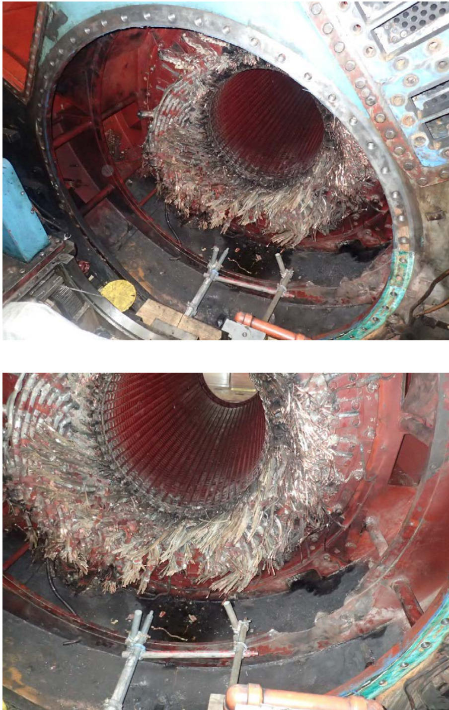
Figure 15. Views of the south (turbine) end of the generator after broken parts, windings, and debris have been cleared out of the machine. Note in the top right corner of the upper image that one of the hydrogen coolers is still in the generator; this cooler could not be removed due to mechanical damage from the failure event.
