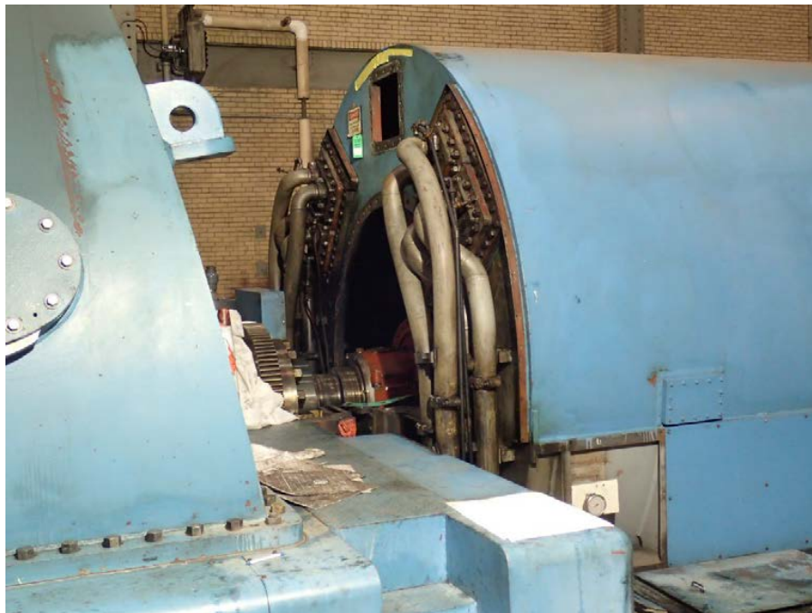
Figure 2. Northwest views of the generator and the damaged end of the generator (lower image) adjacent to the steam turbine. Some components have been removed to permit visual examination of the interior of the generator.
