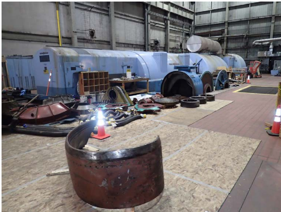
Figure 17. Views of the various components from the generator, temporarily stored on the turbine deck. The lower image also shows the failed retaining ring in the foreground.
