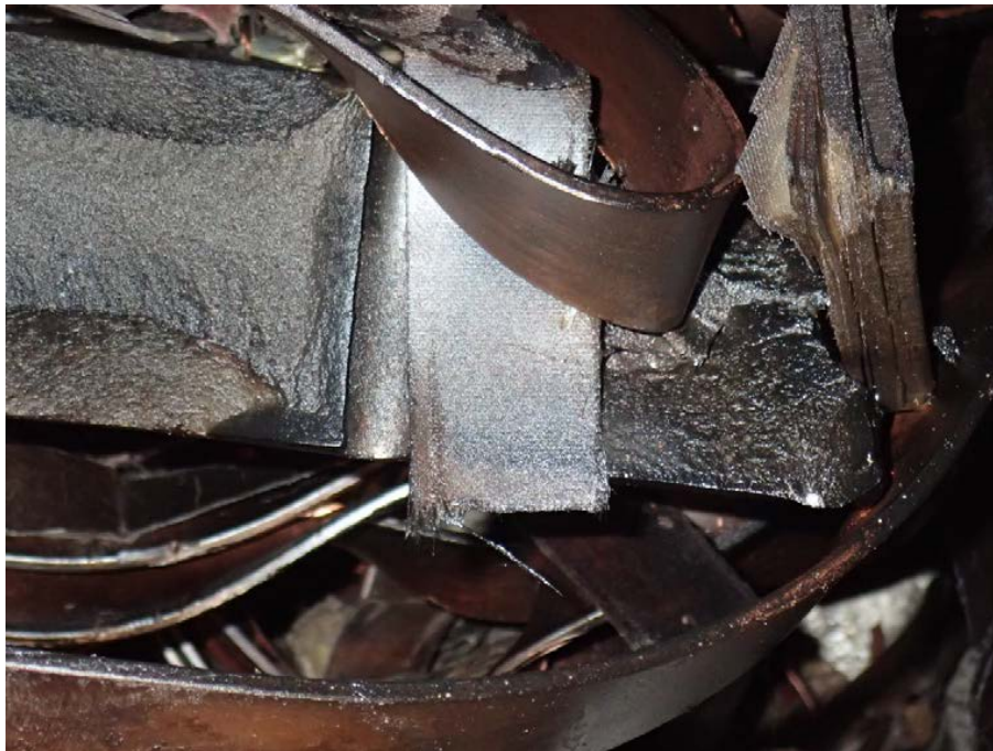
Figure 8. Views of the fracture surface at the lower end of the retaining ring (situated beneath the rotor) (arrow). The lower image is a view of the outboard side of the lower fracture. Debris was blocking clear views of much of the lower fracture surface.
