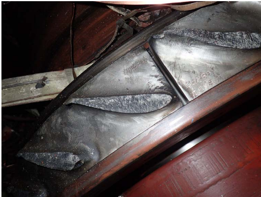
Figure 9. Views of representative blade roots on the hydrogen cooling fan adjacent to the retaining ring.
