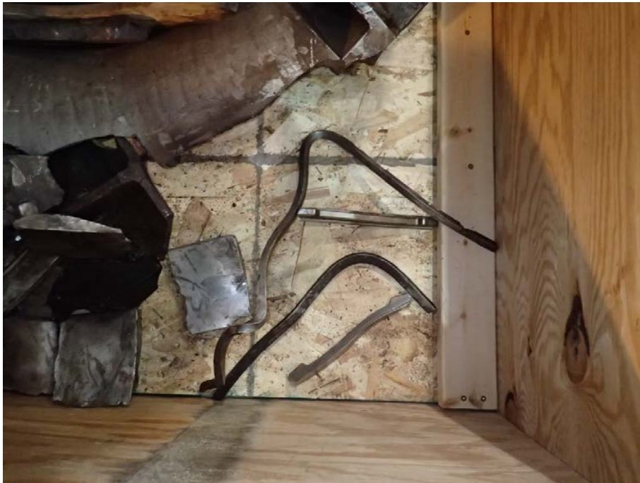
Figure 19. Views of some of the collected debris, which included a snap ring and keys that were associated with the retaining ring at the south end of the generator.
