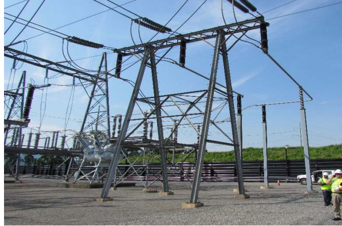
Image 6: Typical A-Frame Deadend Structures
