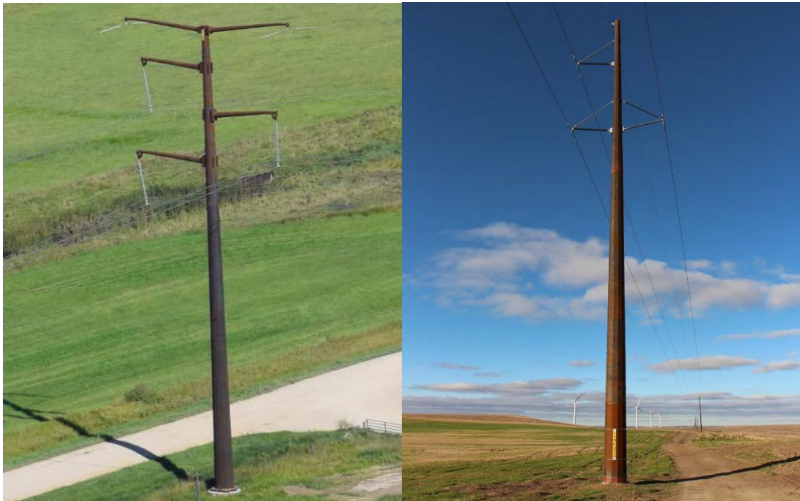
Figure 10. Example of 345 kV Structures
