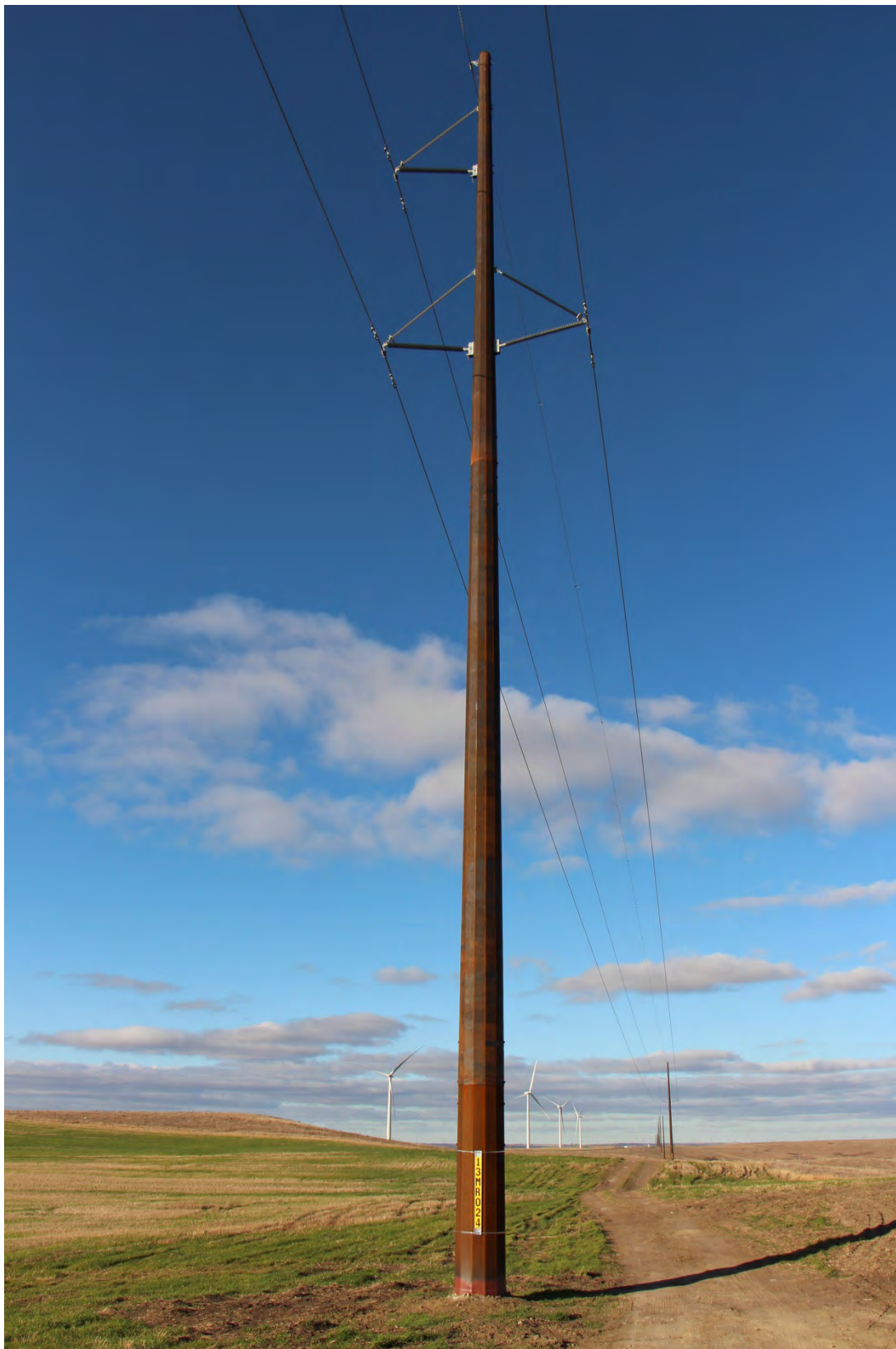
Figure 12: Representative Single-Circuit Structure Sample Photograph
