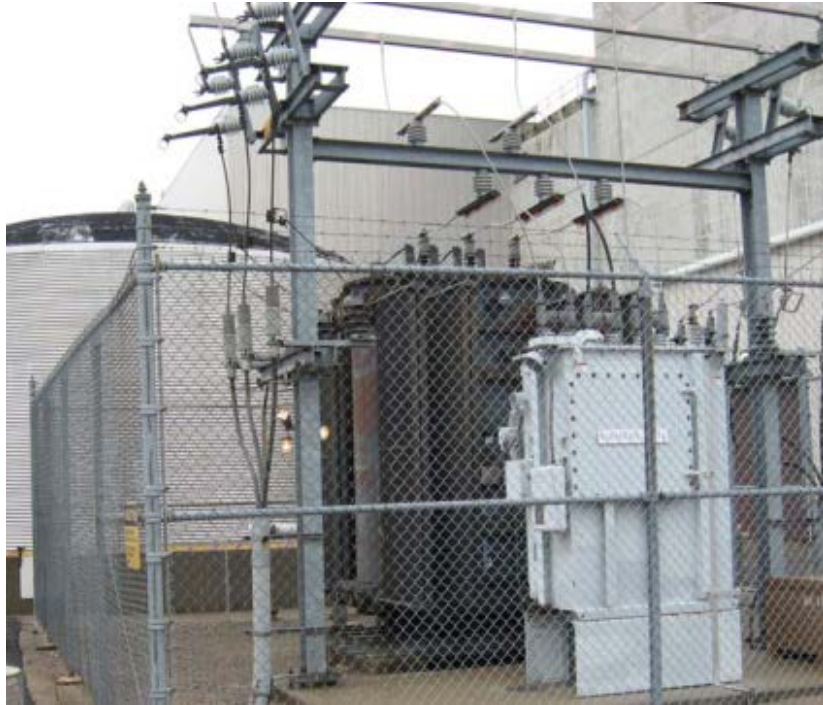
Existing 1AR Transformer Before Removal
