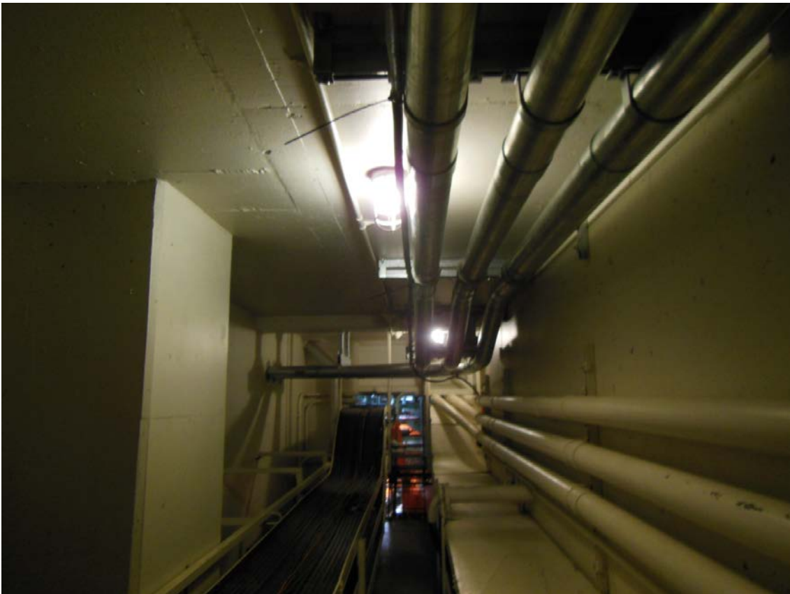
13.8 kV Power and Control Cables in Conduits and Raceways
