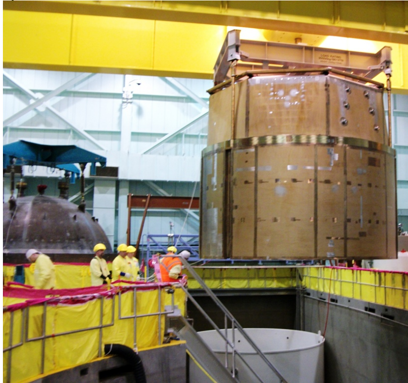
New Steam Dryer Installation
