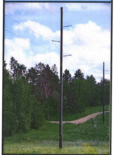
Typical 115 kV Wood Transmission Structure
