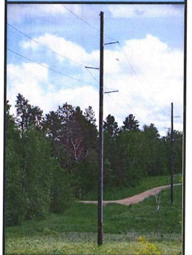
Typical 115 kV Wood Transmission Structure
