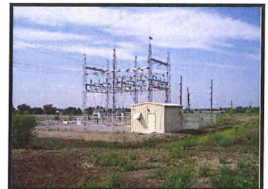
Typical Transmission Breaker Station
