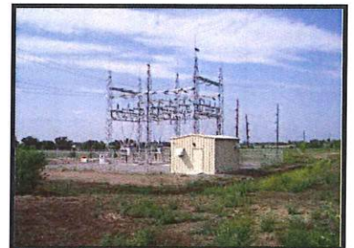
Typical Transmission Breaker Station
