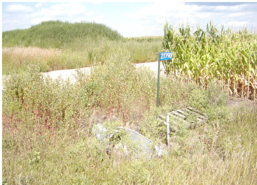
Entrance Drive to Substation Pad w Culvert & RFD Signage
