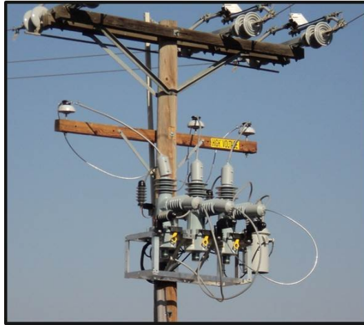
Recloser on Distribution Pole
