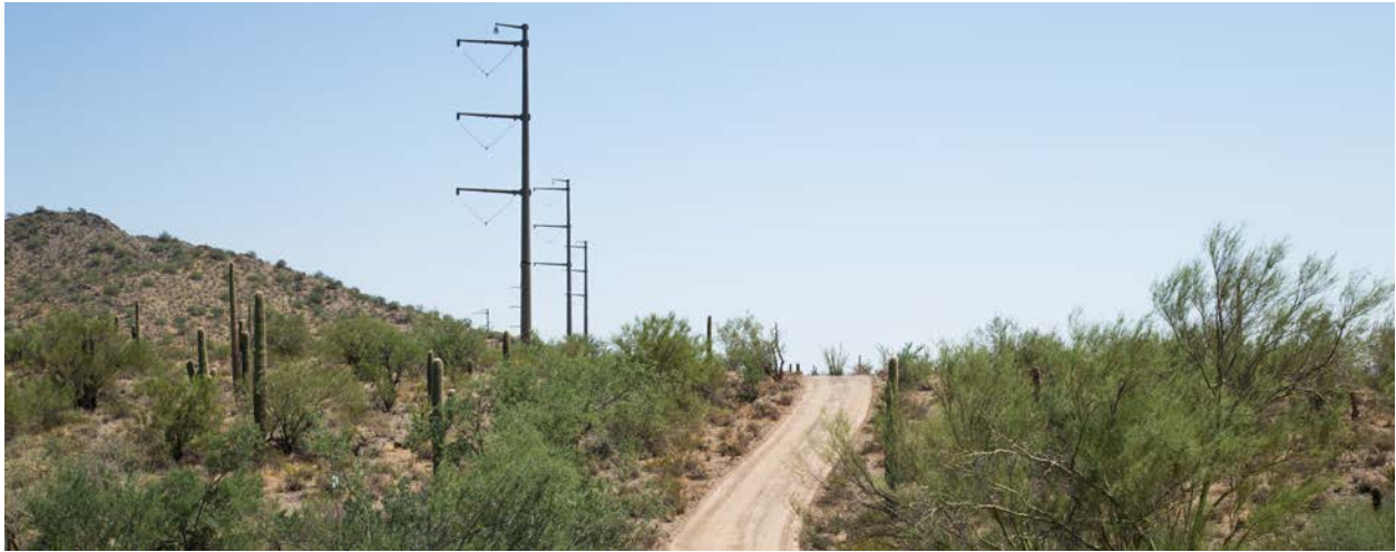
Figure 30 - Powder coated poles back lit
