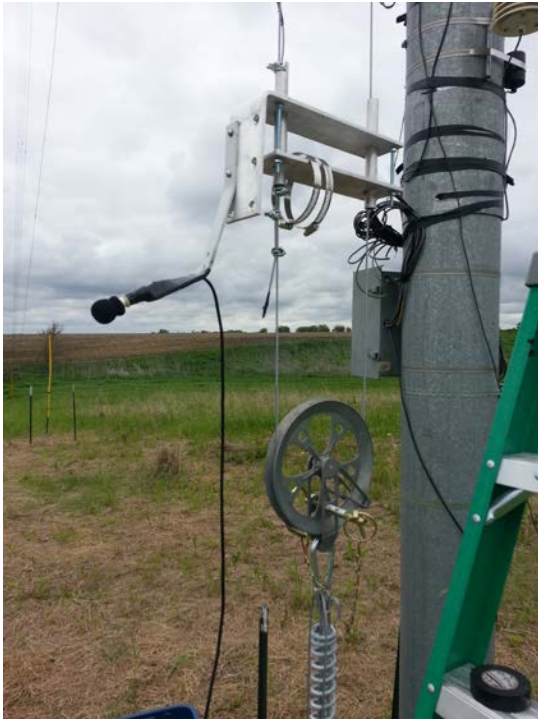
Photo 1. Tower 2 pulley assembly (tower 3 utilizes same system).
