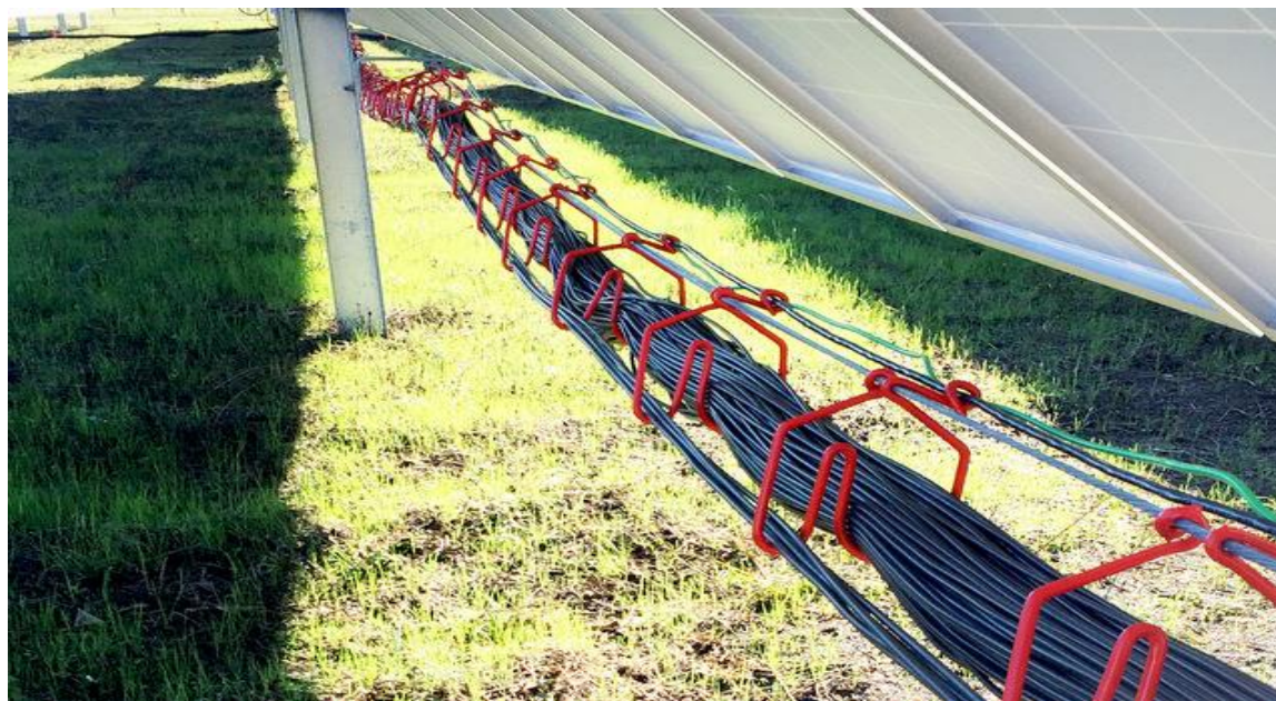
Image 3: Hanging Harness System for DC Cabling between Panels and Inverters
