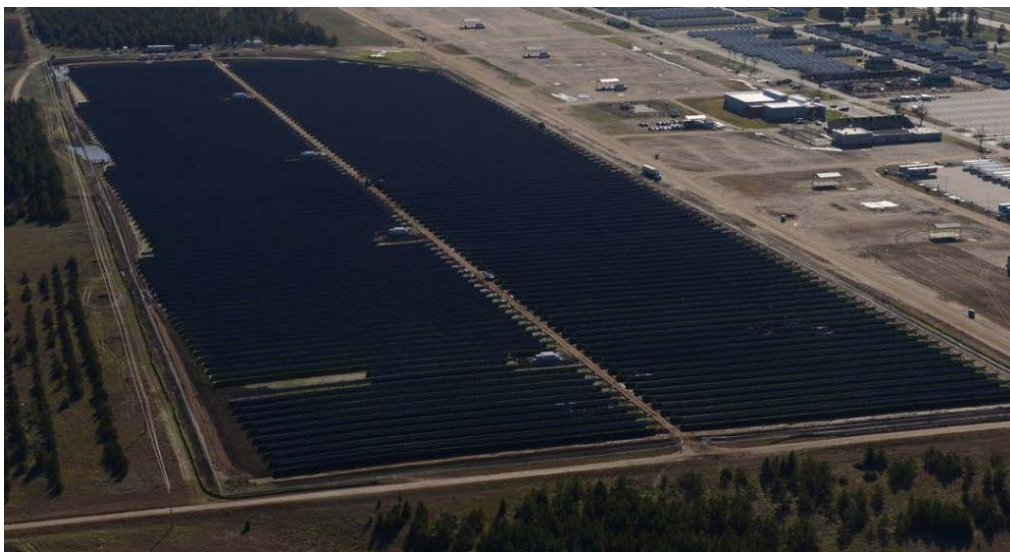
Figure 1- Aerial view of the Camp Ripley Solar Facility
