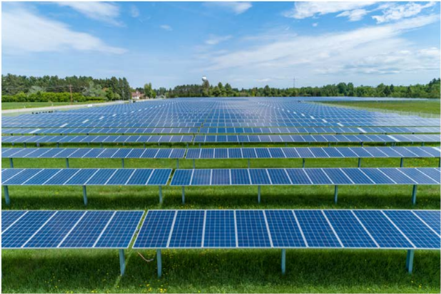
Figure 3- 1 MW CSG Solar Array in Wrenshall, Minnesota
