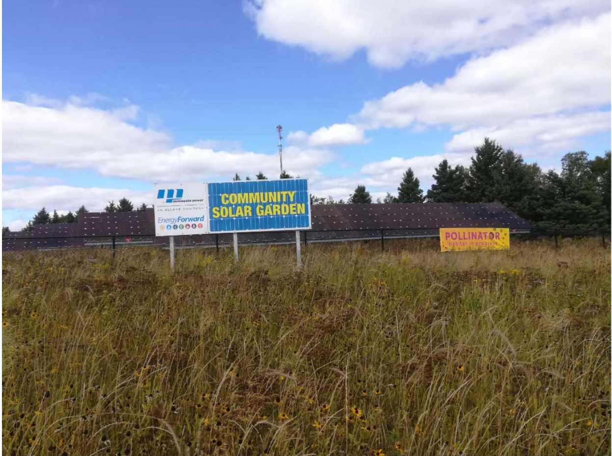
Figure 4- 40 kW CSG Solar Array in Duluth, Minnesota
