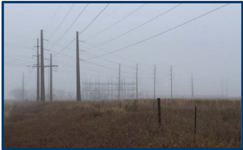
Figure 11 Existing Infrastructure: Glenworth Substation and Other Infrastructure
