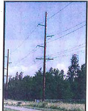
Typical 115 kV Wood Single Circuit Transmission Line Structure with Distribution Underbuild
