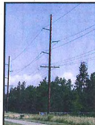
Typical 115 kV Wood Single Circuit Transmission Line Structure with Distribution Underbuild
