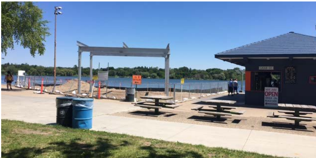
Photo 1: Installation of canopy structure to hold 7.380 kW DC array at Nokomis Park
