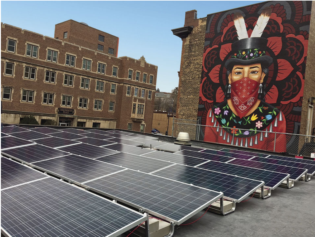
Figure 11: American Indian Community Housing Solar Project
