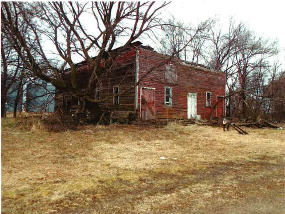
Figure 84. Feature 4, a deteriorating barn, looking to the southwest.
