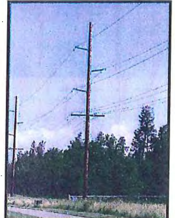
Typical 115 kV Wood Single Circuit Transmission Line Structure with Distribution Underbuild
