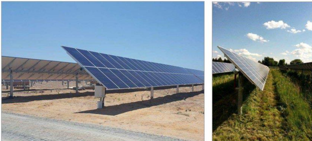
Figure 4. Typical Solar Array
