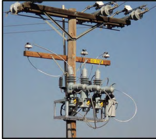
Recloser on Distribution Pole
